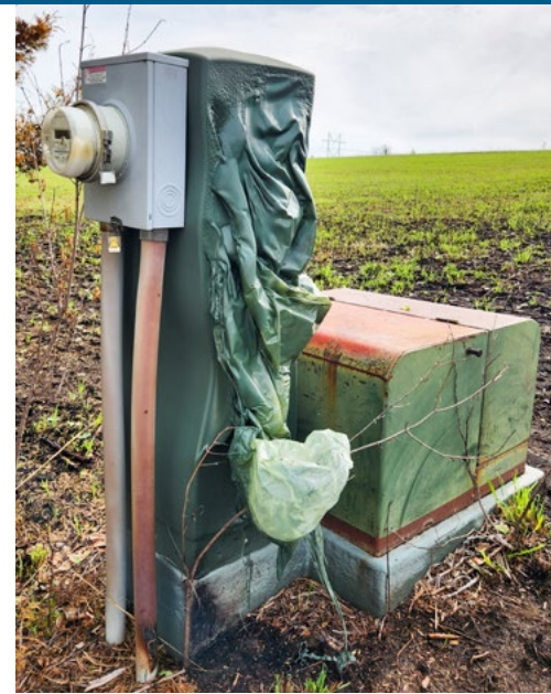
Before burning, check the property for electrical equipment — like this pad-mounted transformer — and power poles to avoid damage and potential outages.
